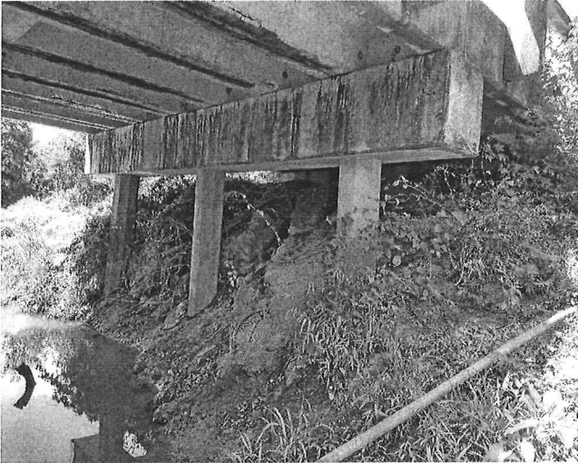
Figure 1. Scour of the west endslope.
