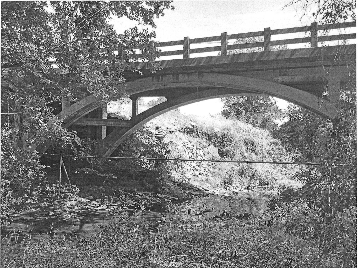
Figure 1. Isabell Creek Cutting into the sandstone and shale bluff on the north bridge end.
