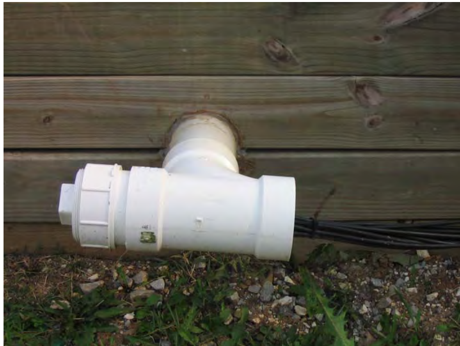
Figure 3.59 Cables of moisture probes went through a PVC pipe, which penetrated through the waterproof retaining wall.
