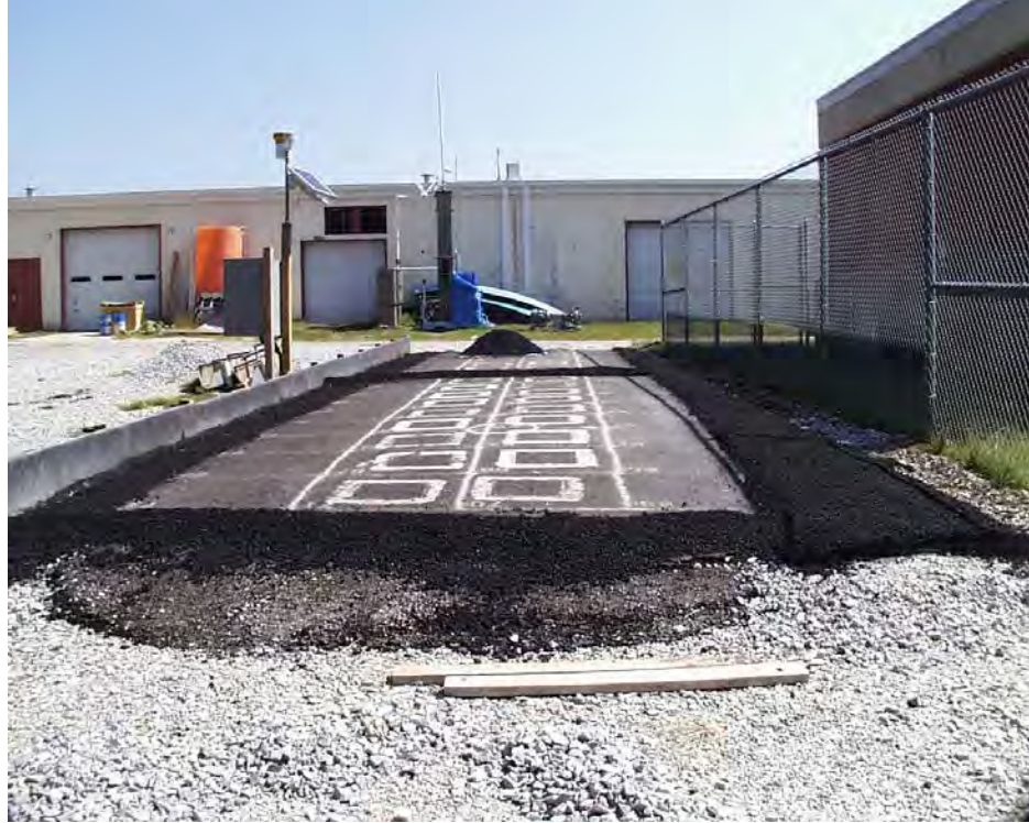
Figure 3.65 Retaining wall and asphalt berms constructed to channel surface water to water flow measuring equipment.
