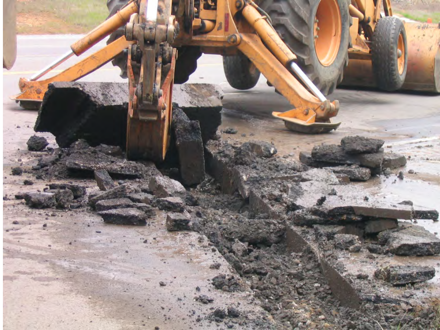
Figure 3.70 Trench excavation for installing moisture and temperature probes at the field test site on Highway 253 in Fort Smith Arkansas.
