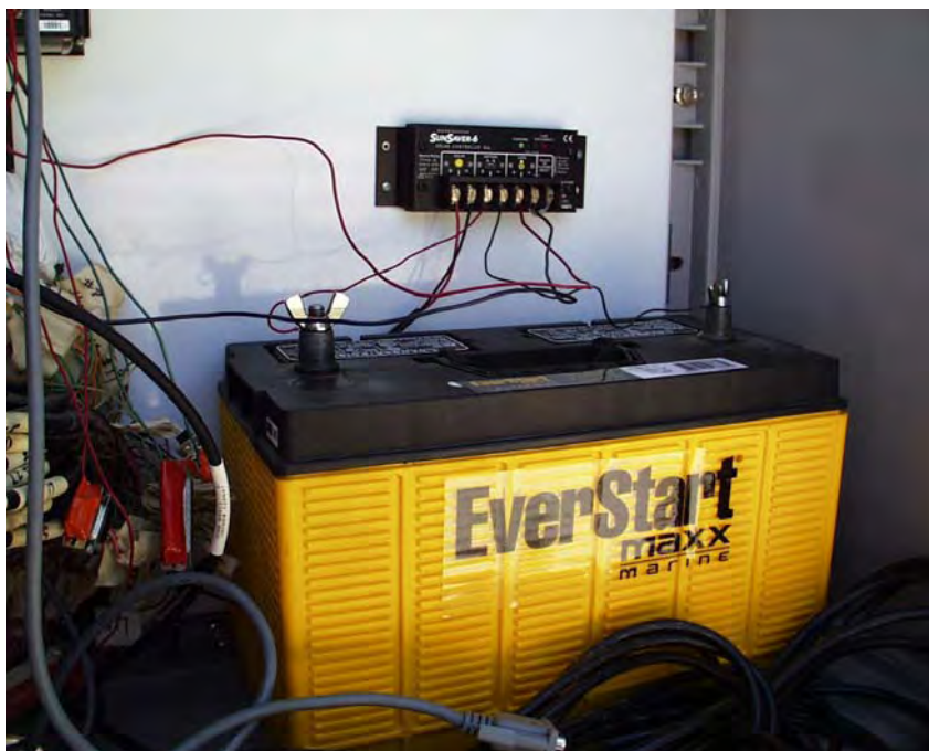
Figure 3.31 Marine battery and controller.
