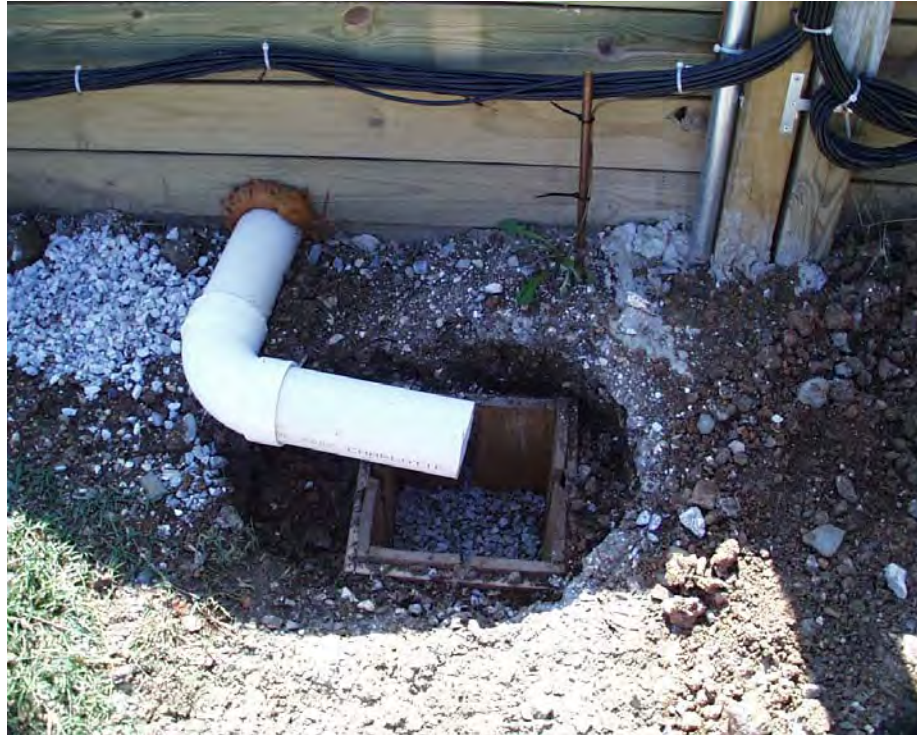
Figure 3.61 One end of a white PVC pipe was connected to the edge drain on the other side of the retaining wall (not shown in this picture), and the other end runs to a wooden box, where a tipping bucket rain gage would be installed.
