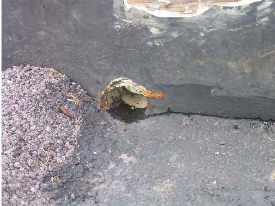
Figure 3.63 A PVC pipe penetrated the waterproof retaining wall and sealed around the contact between the PVC pipe and the retaining wall to channel surface water to flow measuring devices in the other side of the retaining wall, shown in the next figure.
