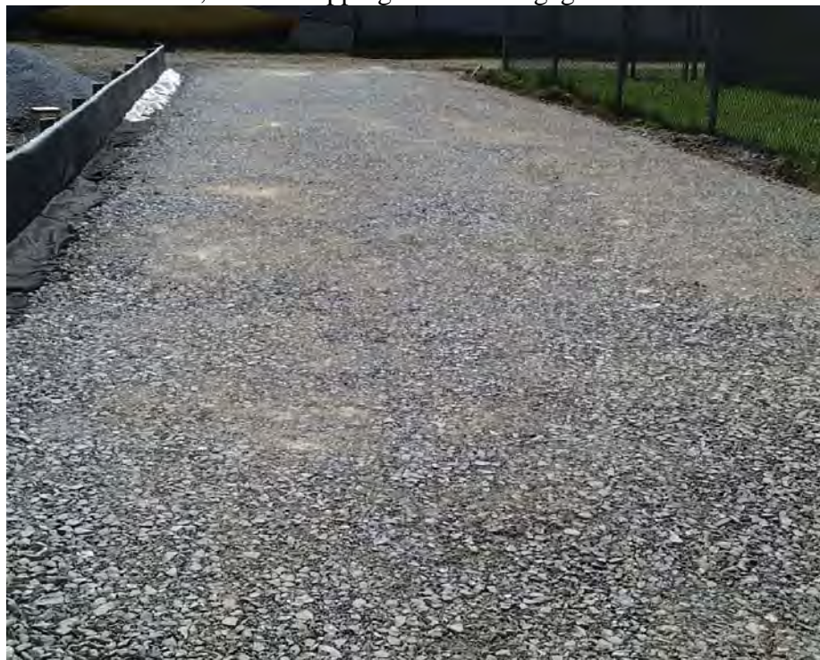
Figure 3.62 Finished base course surface before paving, edge drain wrapped in a geotextile can be seen in the left upper corner.
